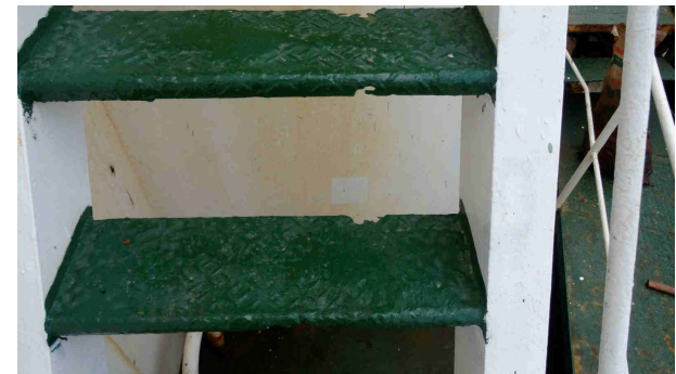
picture 33: the steps are particularly destroyed by rust
