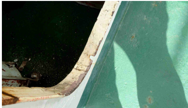
picture 21: door frames were rusted and holed
