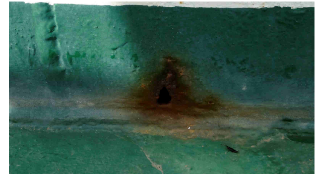
picture 52: several rust-made holes on deck, ...
