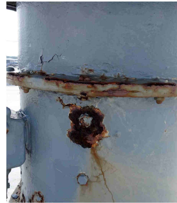
picture 17: not only flange but complete structure rusted
