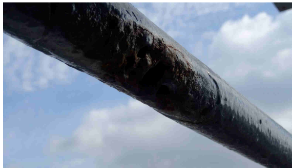
picture 30: holed railing
