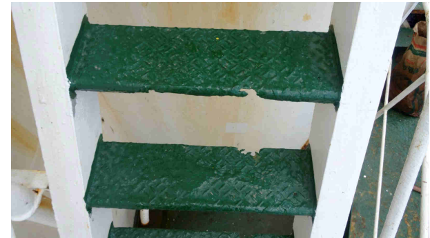
picture 32: in general outside staircase in bad condition
