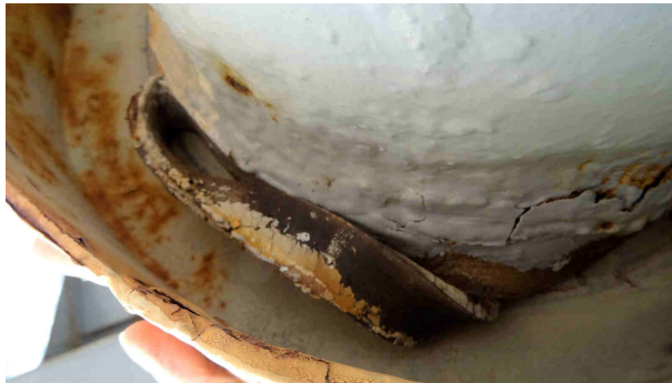
picture 11: damaged rubber on fire damper
