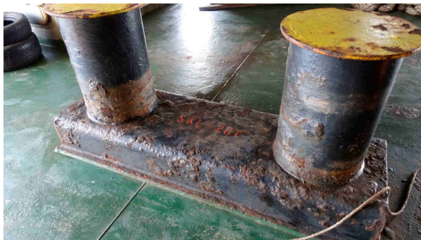
picture 27: bollards with some rust
