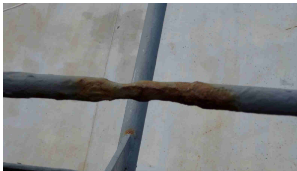
picture 31: what is the name for this condition?
