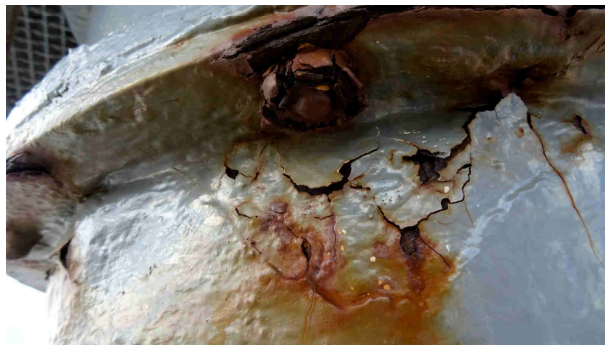
picture 12: corroded flange on fire damper
