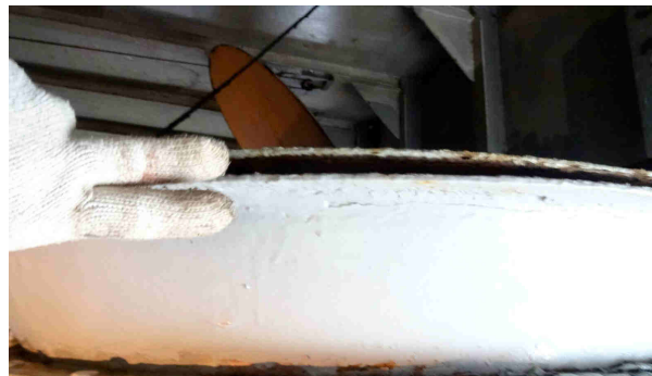
picture 16 ventilation flaps for car decks are not closing properly
