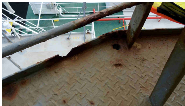
picture 51: general poor condition on platforms
