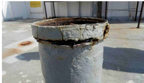
picture 15: next fire damper, same story
