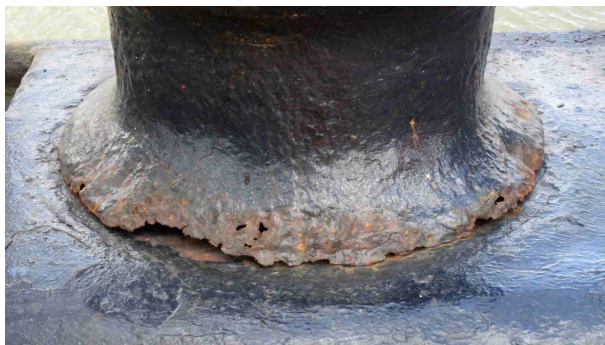
picture 28: capstan damaged by rust
