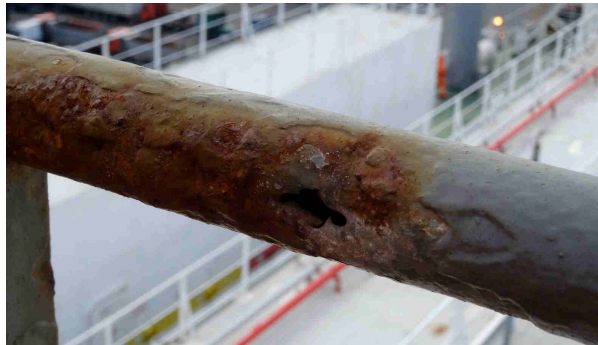
picture 29: rusted railing
