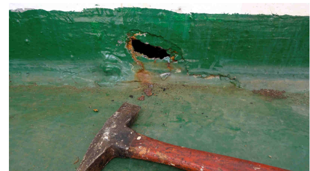
picture 54: additional holes could be made easily
