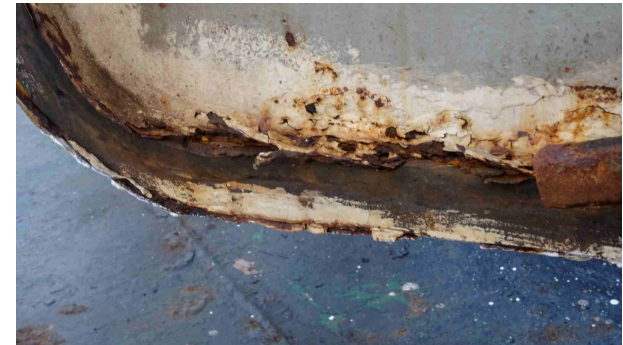
picture 24: corrosion on inner frame on door
